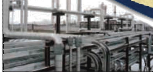
East/West pipetrack showing inlets and outlets to process equipment
